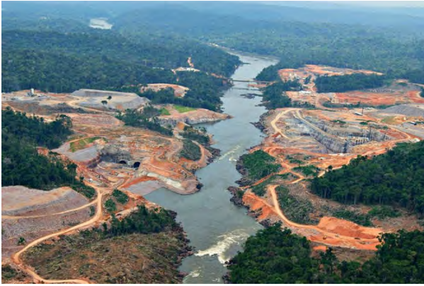
Construction of the São Manoel Dam in the Brazilian Amazon. International Rivers/Flickr, CC BY-NC-SA
